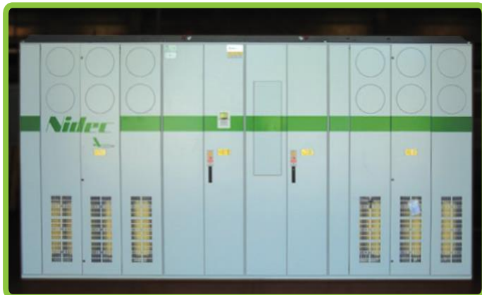
"Flumeri 1.2MW" PCS – DC/DC секция (CHOPPER)
