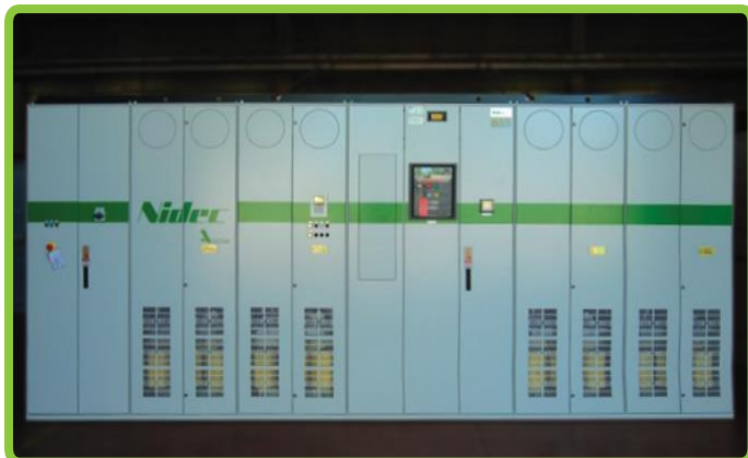
"Flumeri 1.2MW" PCS – AC/DC секция (AFE)
